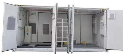
1075KW HH ESS
