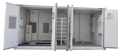
1075KW HH ESS
