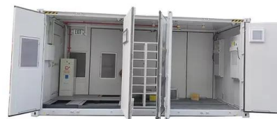
1075KW HH ESS
