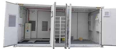
1075KW HH ESS
