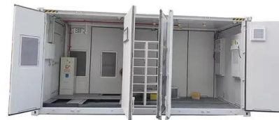
1075KW HH ESS
