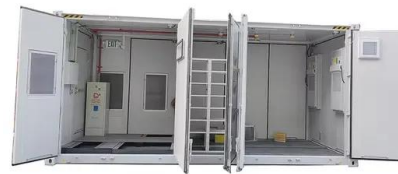
1075KW HH ESS
